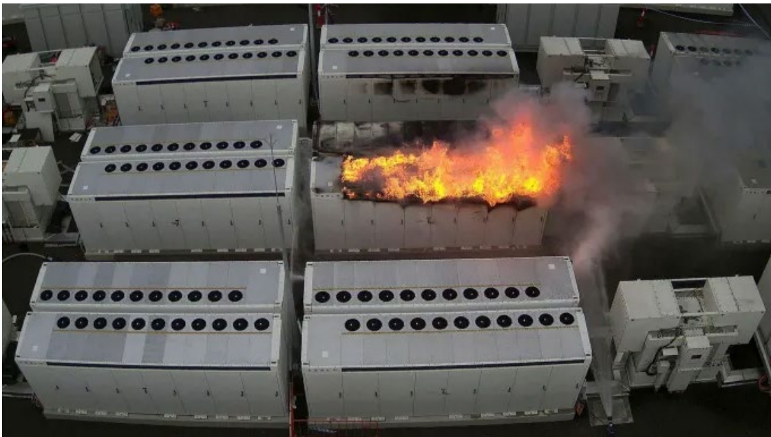
Figure 2. Thermal Runaway Fire on a Battery Pack
